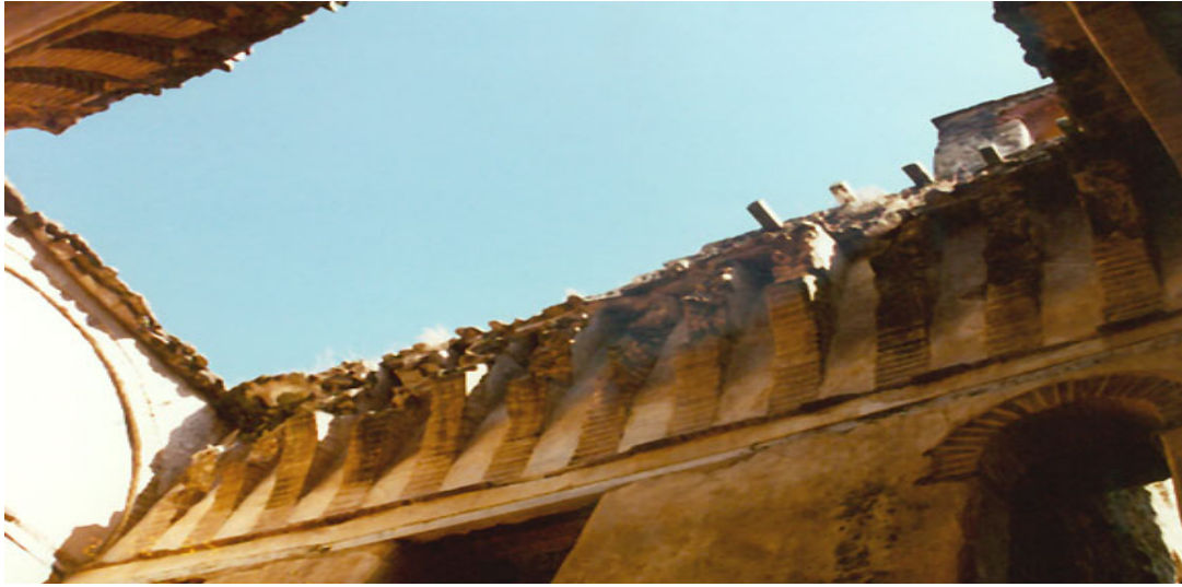
Figure 3-Similar Room where the Ceiling has fallen
